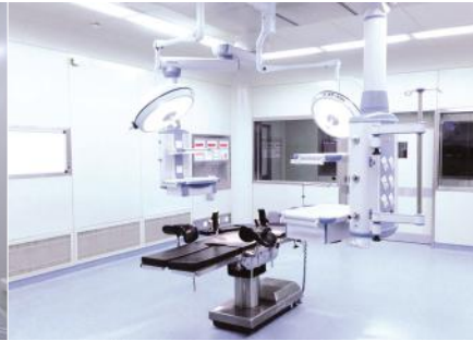
Integrated purification for operating room
